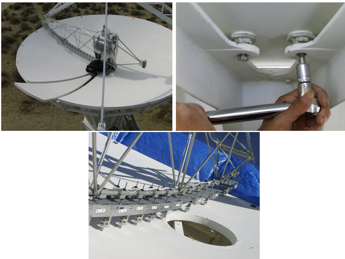
Figure 2.3: Surface setting campaign. Top left: photo taken during installation of a previously unused panel. Top right: reattachment of panel to telescope support after shim thickness had been changed. Bottom: close-up of the measurement arm and capacitive sensors; panel in photo was later replaced.
